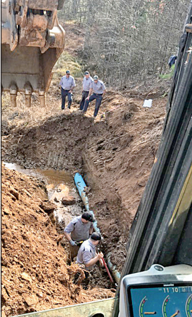
The 12-inch water main break occurred behind The Sanctuary at Lake Nottely on Murphy Highway
